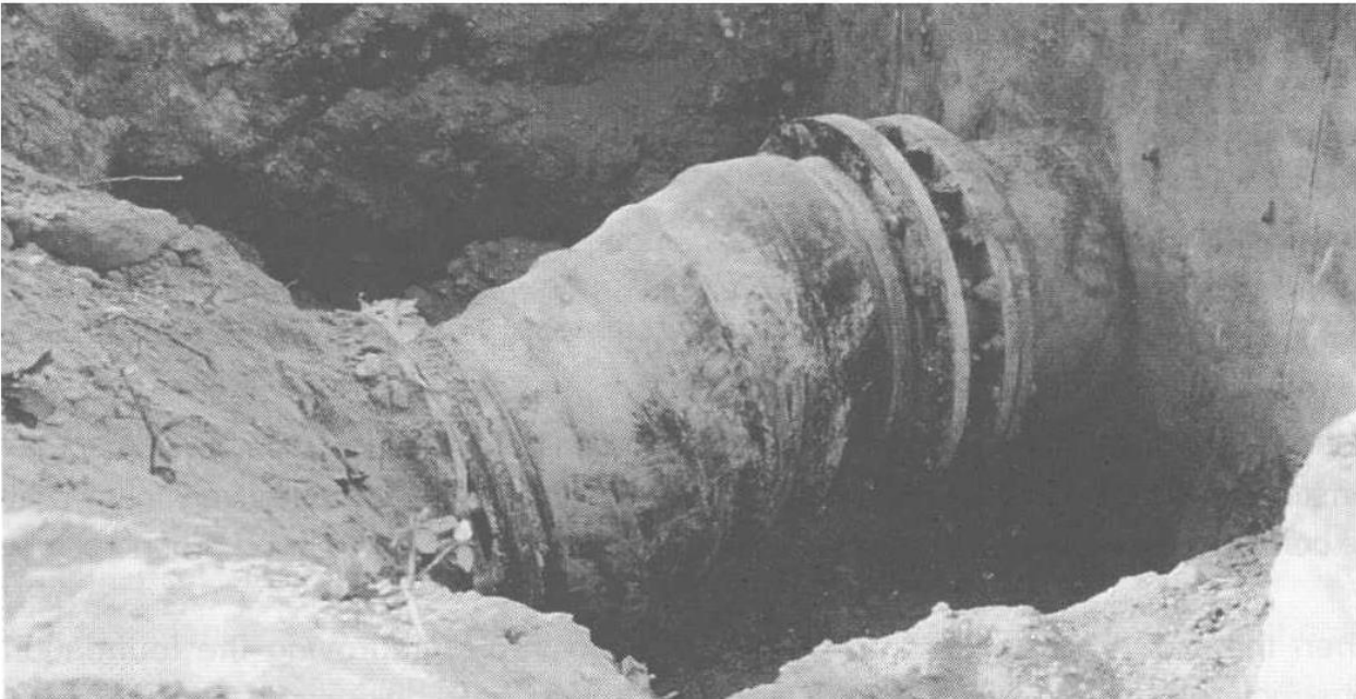
Figure 10 Deformed flexible pipe (Kobe-Japan)
